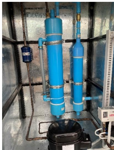
Fig. 8 Complete scrubbing and gas compressor for biogas in OTOP Duang Thong District
