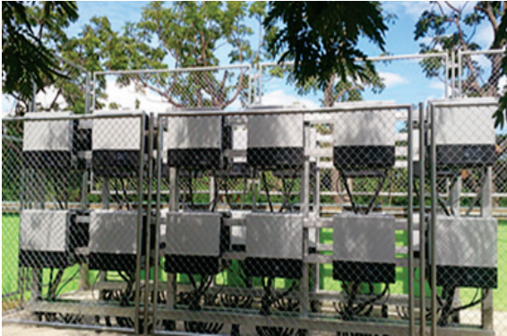
Figure 3 Installed inverter in Mukdahan.
